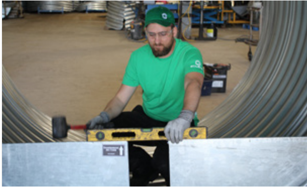
7c. Using the hammer or rubber mass, make sure the weir is level. Soleno recommends wearing hearing protection.
