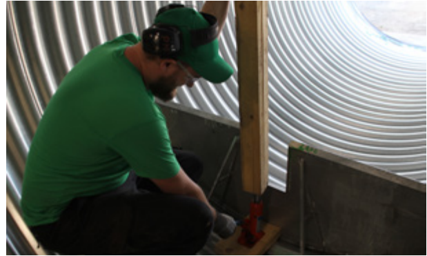
7d. Using the jack and the wooden adapter, hold the weir at the bottom of the culvert.
